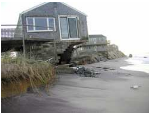
Several houses on Nantucket Island were severely damaged by the coastal flooding. [David Gray, Sr, W1ACK, Photo]
